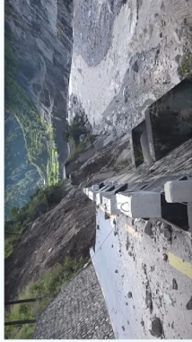
Slope failure at Sindhuli Road, Rosi Khola area
