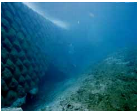
Photo showing scouring of the foundation of a dam
