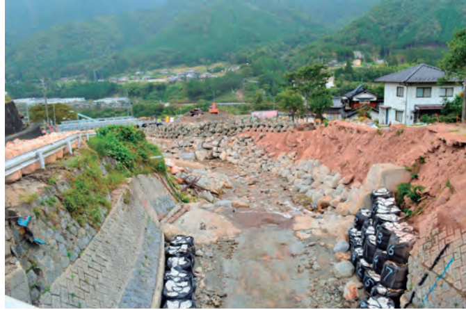
Figure 2. Sand bag and tetrapod as temporary countermeasures placed in riverbank to prevent the debris hit the housing resident. One child was dead when the debris hit his house on July 9, 2014.
