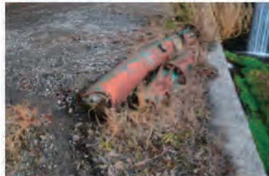
Figure 19 Broken Part of Sabo Dam
