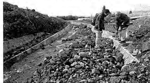
Photo 4 Gravels shown accumulated in the downstream section
